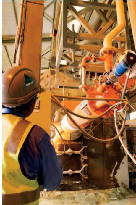
New burner installation on Kiln 3 at Angaston
