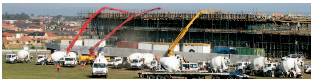
Hy-Tec's geographical spread of concrete plants in Sydney provides the flexibility to utilise supply from a number of concrete plants for large scale concrete pours.
