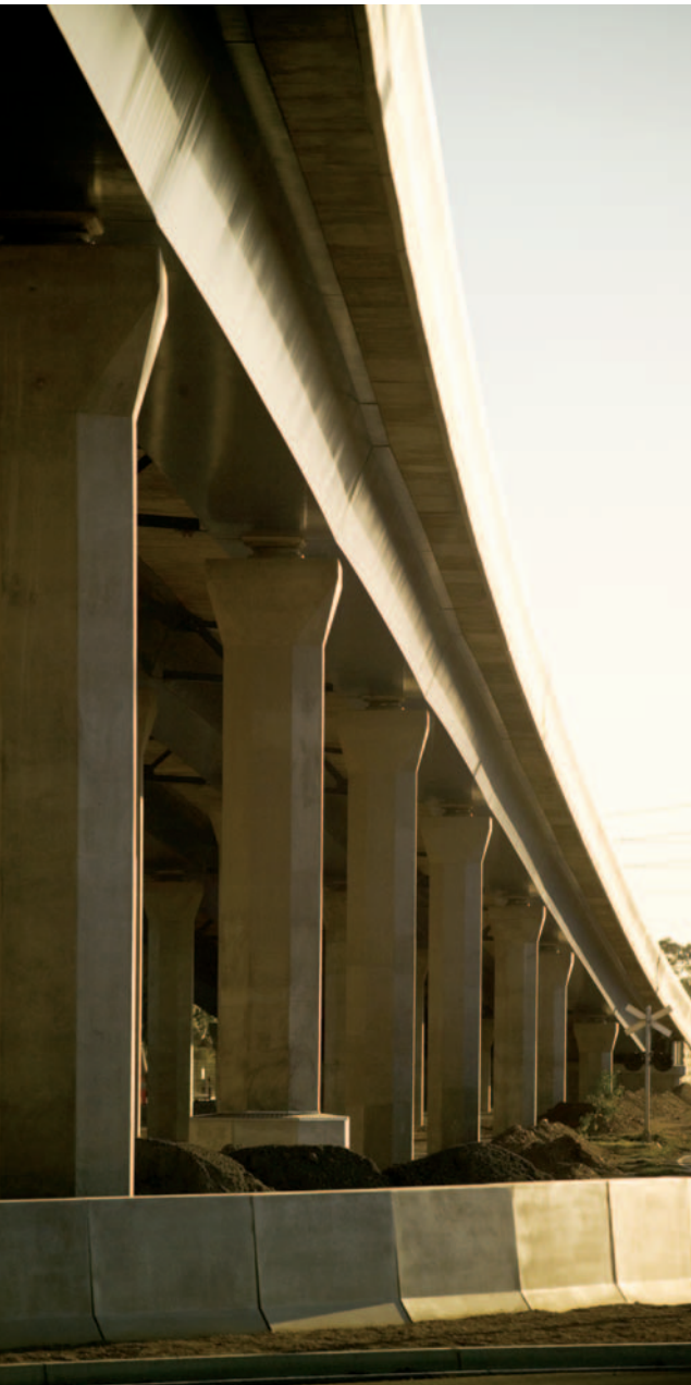
Port River Expressway Eastern Parade Bridge - part of the South Australian Government infrastructure development plan for Port Adelaide. The 270 metre bridge has been constructed using box steel girder beams supported by reinforced concrete columns and an insitu concrete deck slab.
